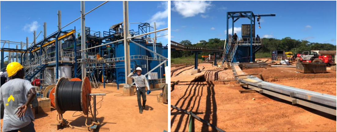
PHOTOS OF THE DIEU MERCI CYANIDATION PLANT AT THE END OF ITS COLD COMMISSIONING 1 PHASE (WEDNESDAY 24 OCTOBER 2018)
