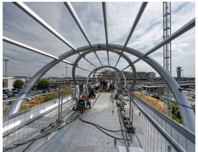
View of the interior of the footbridge under construction ©Groupe ADP - Alain Leduc
