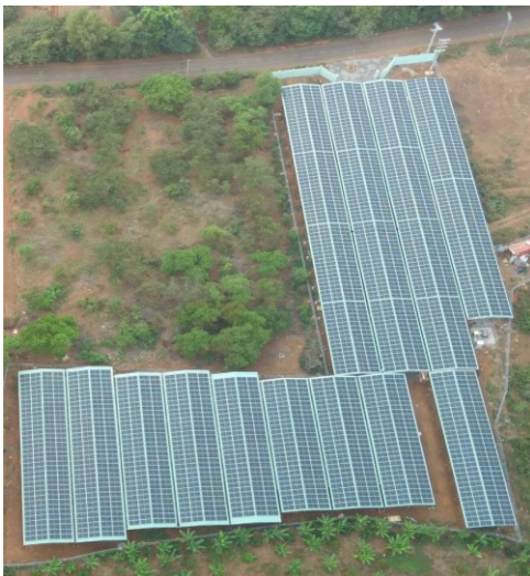
900 kWp solar-power installation on a Vietnamese mushroom farm monitored and managed with LoRaWAN technology.
