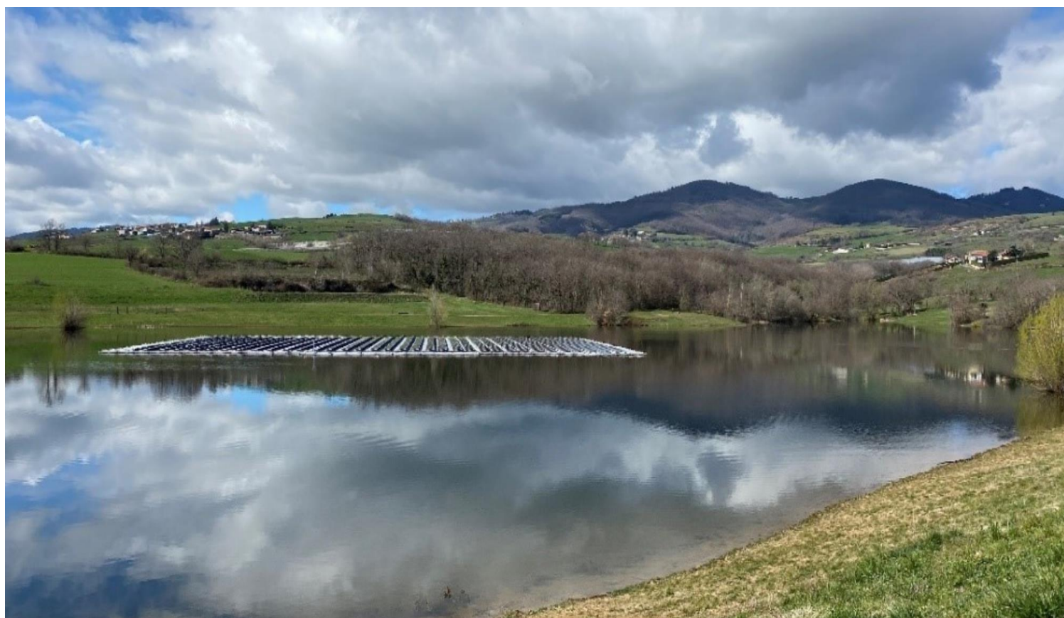
CNR's first floating photovoltaic park (Compagnie Nationale du Rhône)
