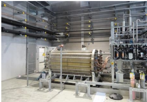
Photo of the electrolyzer after the incident
